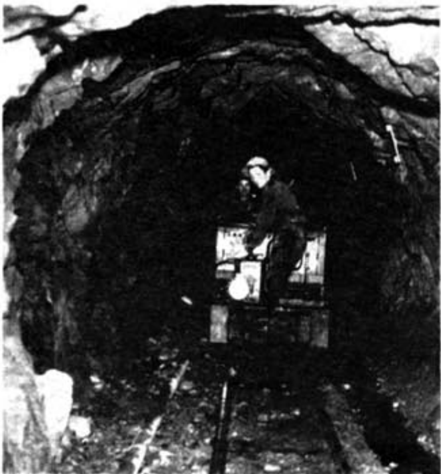
Bridgeport Hydraulic Company workers tunneled 7,100 feet below the solid rock of Popp's Mountain on the Easton-Weston town line to connect the Saugatuck and Aspetuck reservoirs in the 1930s and 1940s. Courtesy of Bridgeport Hydraulic Company.
