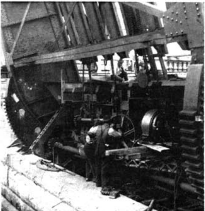
Crew at work on the huge gears of the old Stratford Avenue draw-bridge in 1917.
